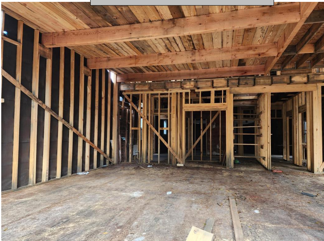
Right Rear Elevation. Window Openings Removed
