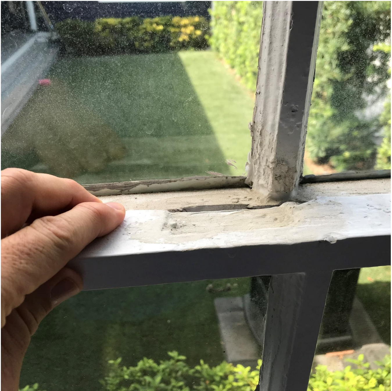
Figure 7 - lower portion of upper sash muntin significant damage
