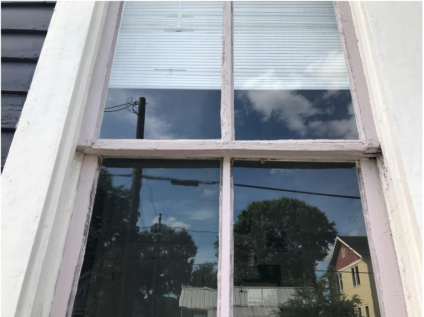
Figure 4 - Upper sash meeting rail needs replacement, lower portion of sash sides and middle muntin need significant repairs.
