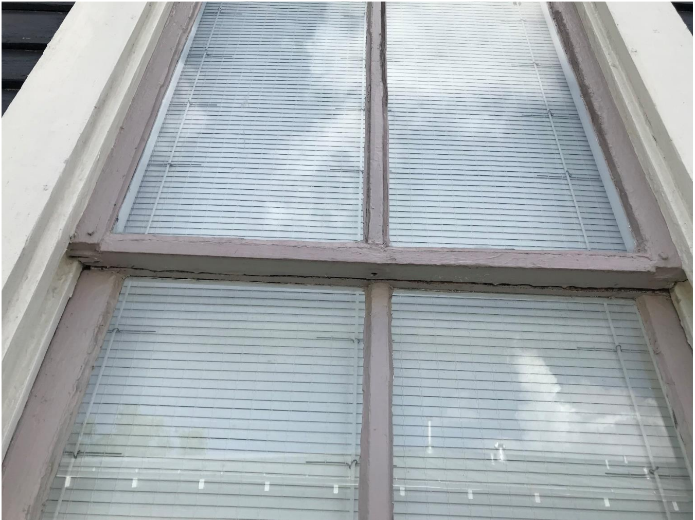
Figure 5 - Upper sash meeting rail needs replacement, lower portion of sash sides and middle muntin need significant repairs
