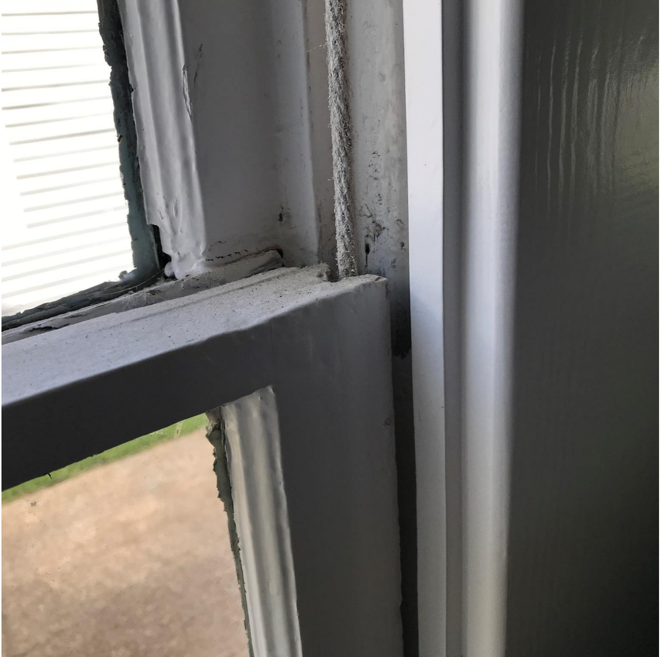
Figure 8 - meeting rails and side rails need replacement or significant repairs.
