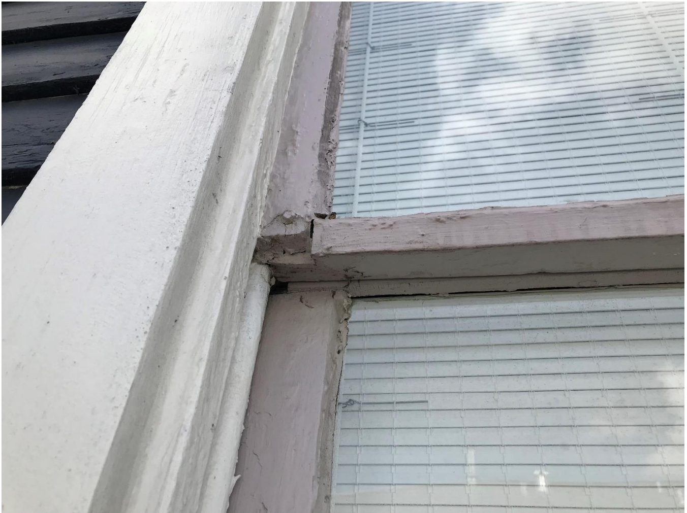
Figure 6 - Meeting rails need replacement, side rails upper and lower significantly damaged
