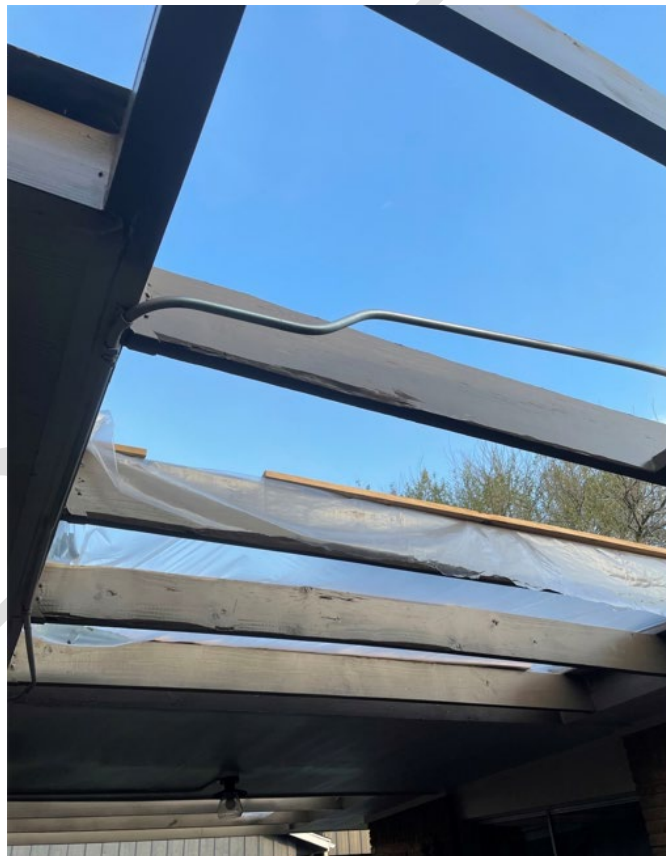
Previously covered roof – open now causes damage to front door and sliding door
