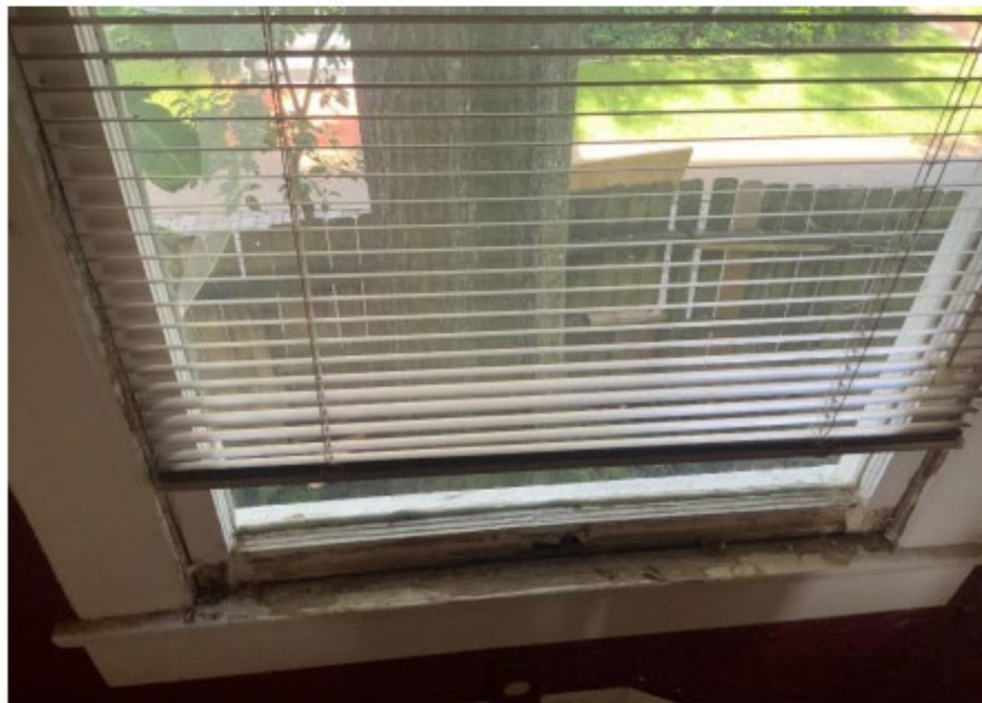
Figure 7 WINDOW B2: Rotten Frame
