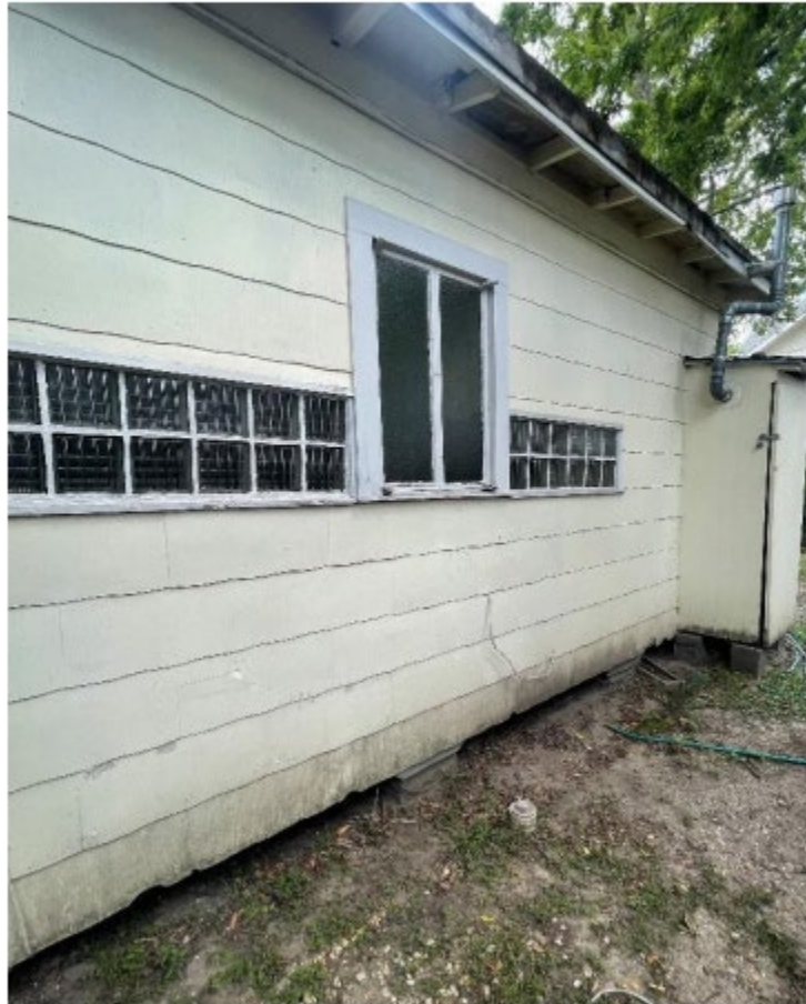
Figure 14 WINDOW H: Not original window to be removed.
