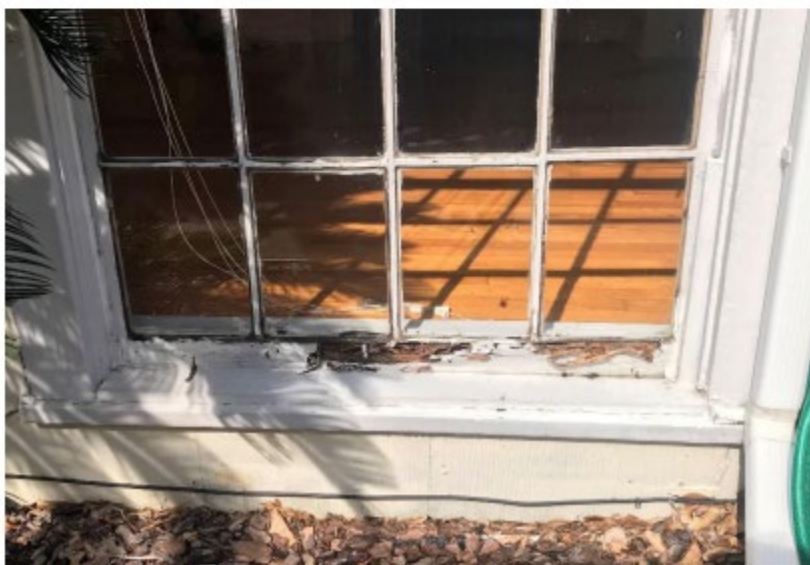
Figure 9 WINDOW F1: Rotten Frame
