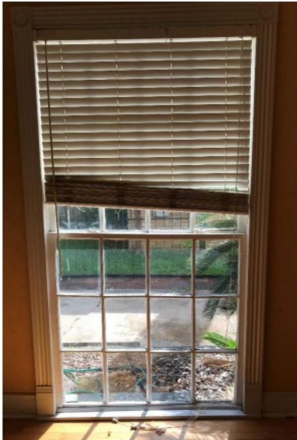
Figure 8 WINDOW F1: Window is inoperable, frame is rotten
