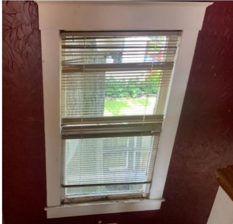
Figure 6 WINDOW B2: Glass is broken, window is inoperable, and frame is broken
