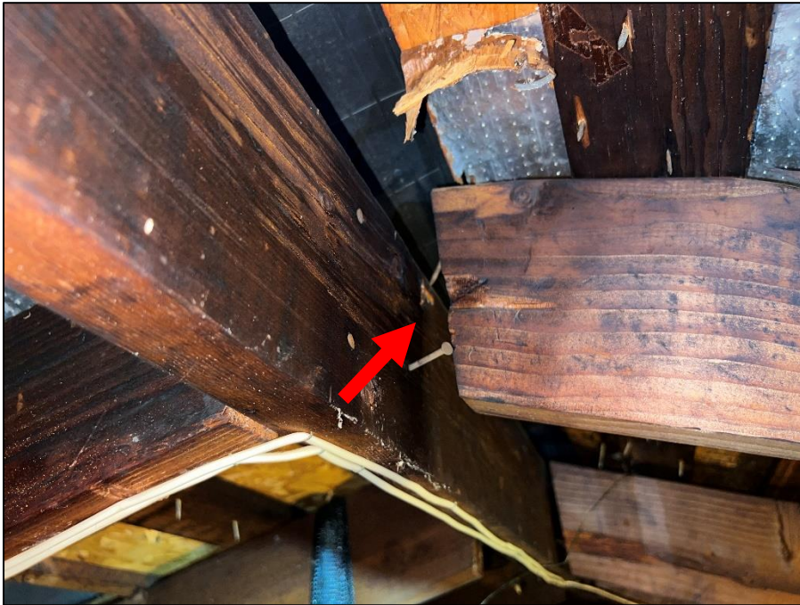
Photograph 40 : Typical view of roof rafters that have been detached from the ridge board.
