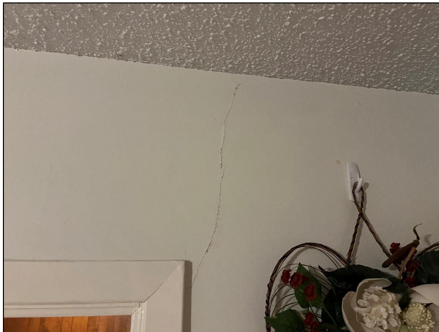
Photograph 30: Typical view of interior wall of the center bedroom ( adjacent to bedroom closet ) displaying drywall cracking extending from the door header.
