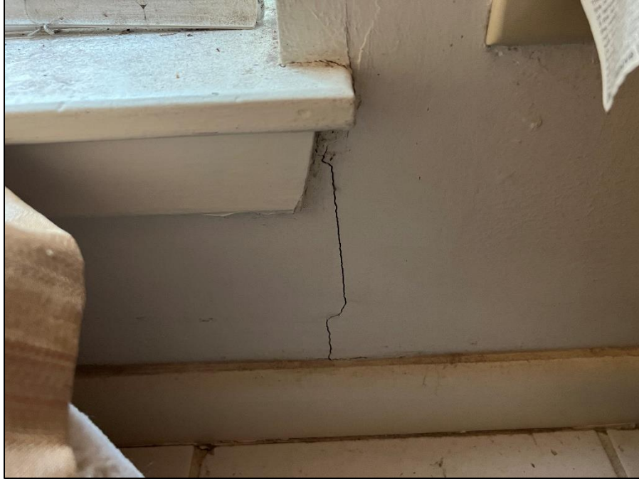
Photograph 25: Typical view of front exterior wall of the front left bedroom displaying drywall cracking extending from the windowsill.
