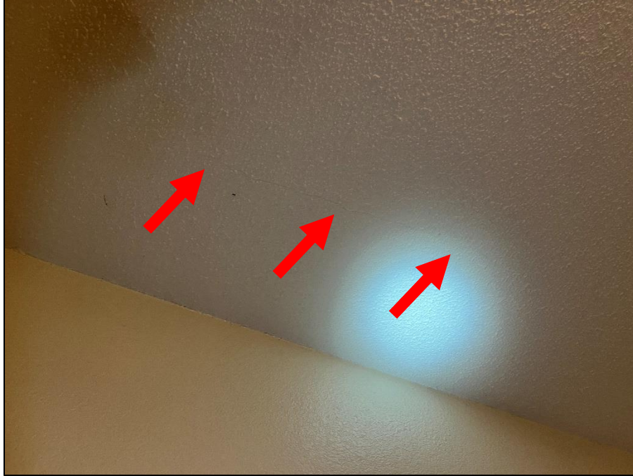
Photograph 19: Typical view of ceiling displaying drywall cracking in the foyer.
