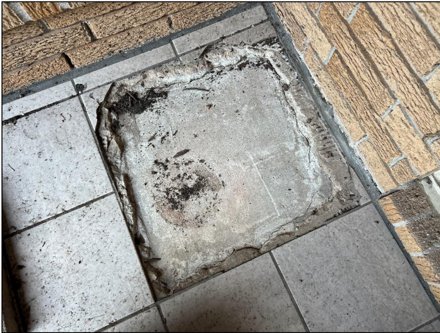
Photograph 8: Typical view of patched concrete flatwork indicating historical foundation repairs/leveling.
