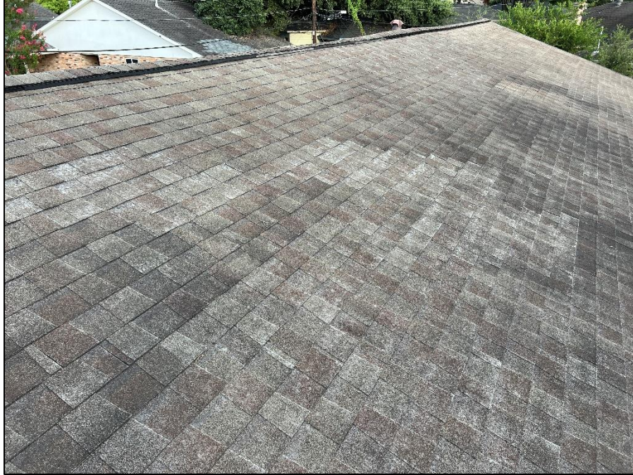
Photograph 45: Typical view of asphalt roof shingles displaying a loss of surface granules.
