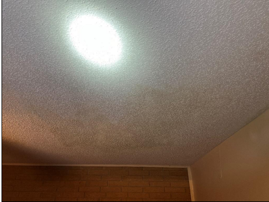
Photograph 31: Typical view of ceiling displaying moisture staining in the center bedroom.
