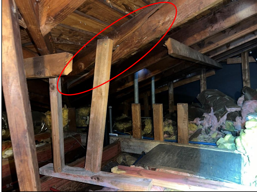
Photograph 41: Overview of roof and ceiling framing within the attic space at the front left of the residence. Notice the broken roof rafter where a two-by-four was installed as temporary support. Also, notice the lack of rafter and purlin bracing within the rafters.
