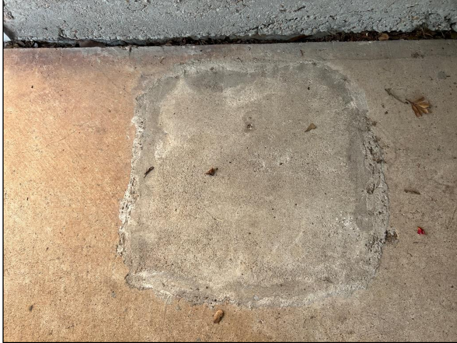
Photograph 11: Typical view of patched concrete flatwork indicating historical foundation repairs/leveling.
