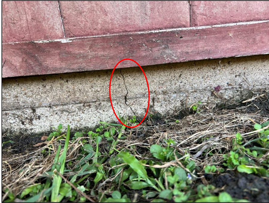
Photograph 17: Typical view of cracking on the exterior perimeter foundation grade beams at the rear of the residence.
