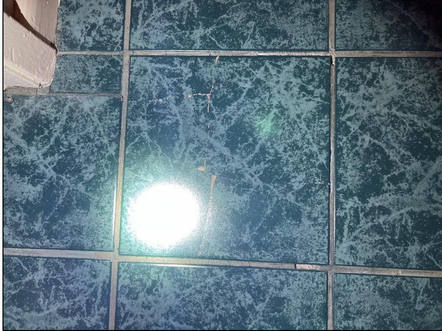
Photograph 23: Typical view of loose tile and cracking within the tile flooring.
