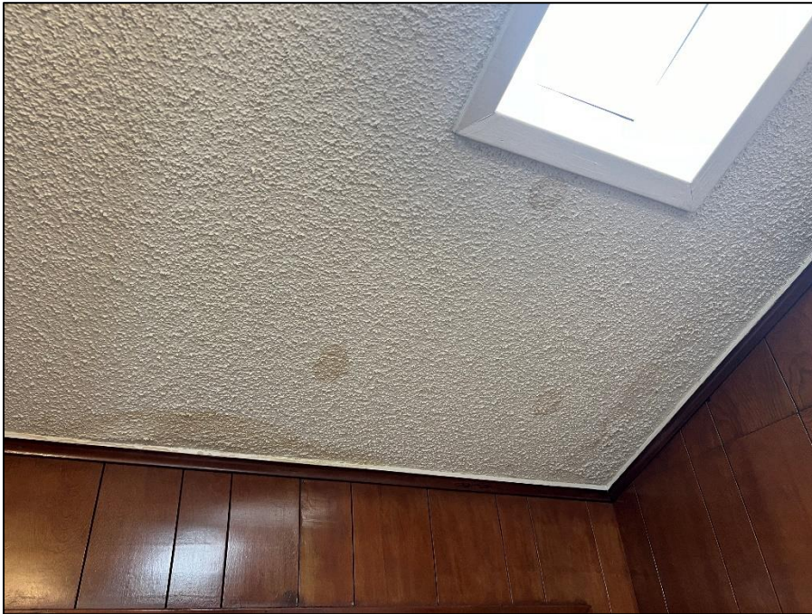
Photograph 34: Typical view of ceiling displaying moisture staining in the living room.
