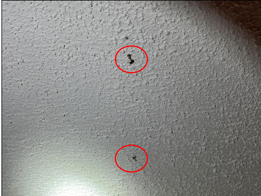
Photograph 37: Observation of ceiling displaying nail pops within the drywall.
