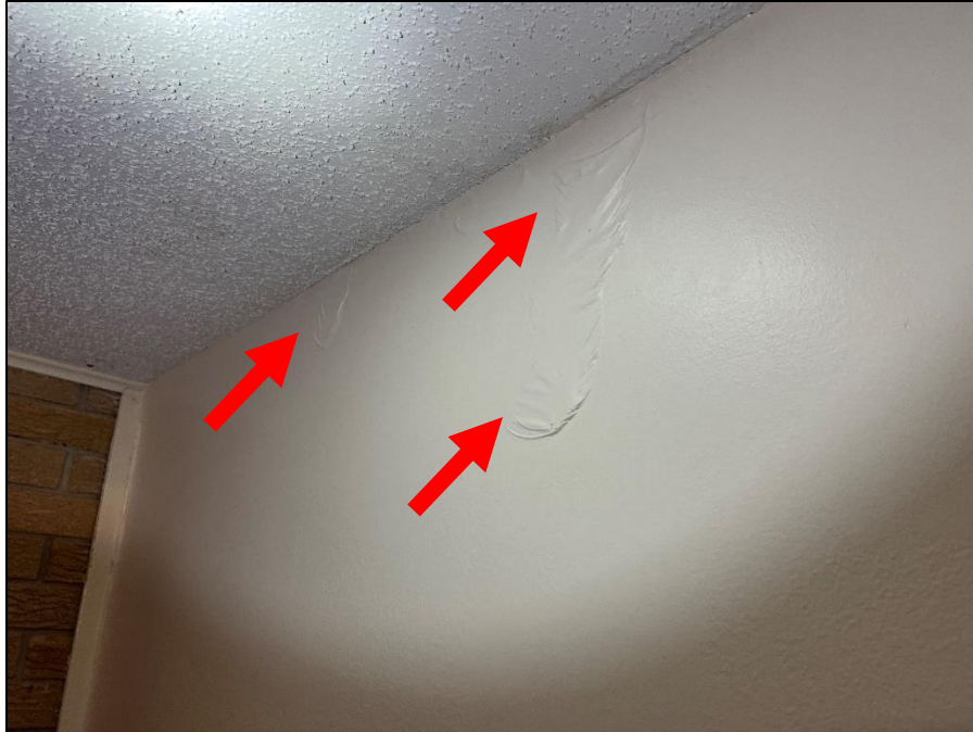
Photograph 29: Typical view of interior wall of the center bedroom ( adjacent to hallway ) displaying wrinkling and/or blistering paint.
