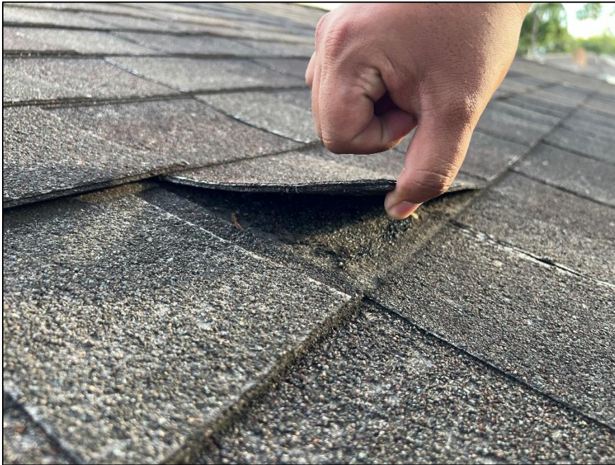
Photograph 44: Typical view of aged and deteriorated asphalt shingles on roof. Most shingles lacked a viable adhesive strip that would keep the overlying shingle bonded to the underlying shingle.
