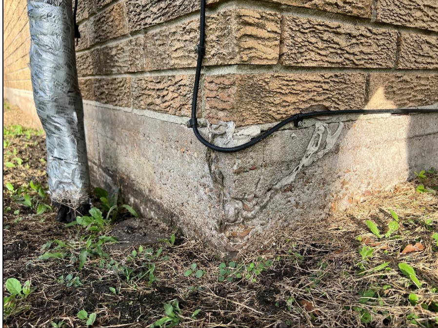
Photograph 5: Observation of foundation concrete corner cracking located at the front left of the residence.
