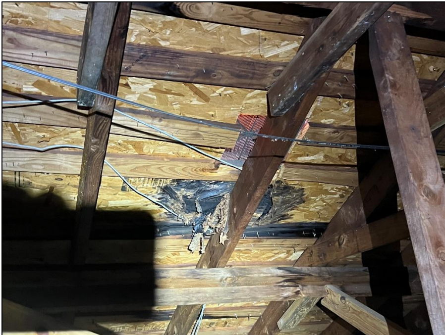
Photograph 42: Observation of roof decking decay indicating historical roof leaks.
