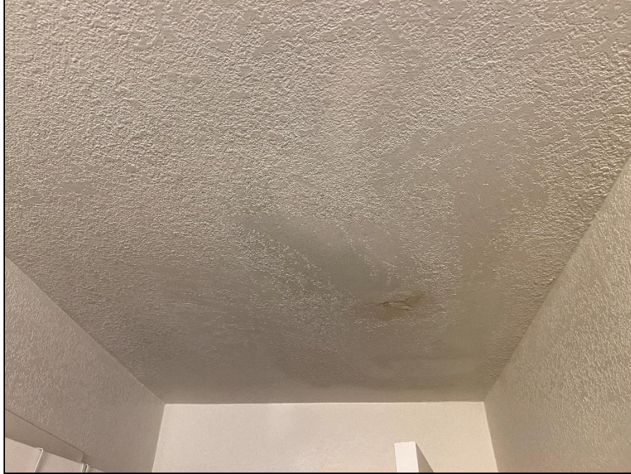
Photograph 33: Typical view of historical drywall ceiling repair.
