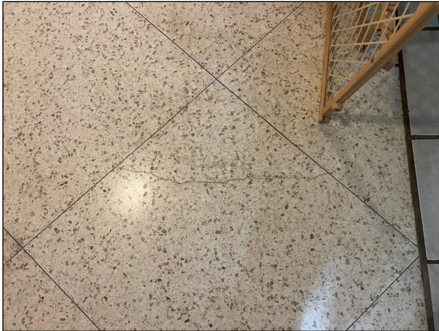
Photograph 20: Typical view of cracking within the terrazzo floor tile.
