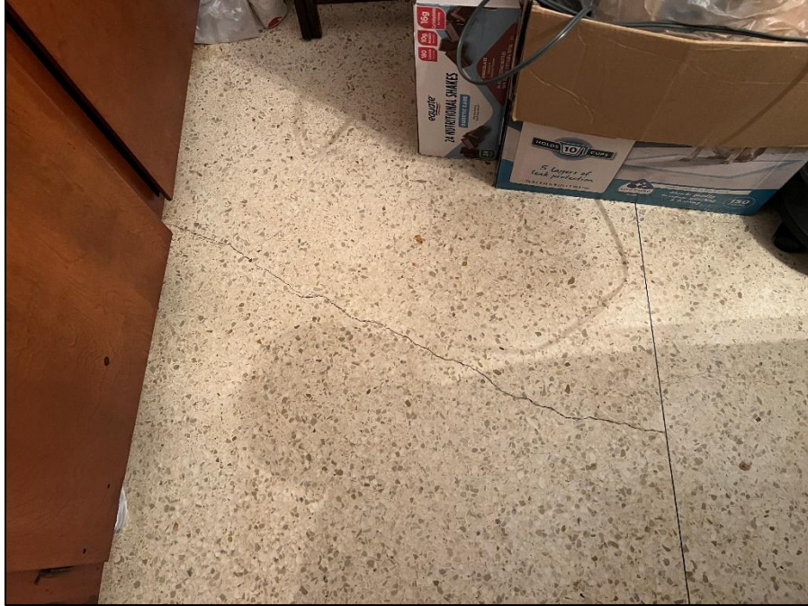
Photograph 35: Typical view of cracking within the terrazzo floor tile.
