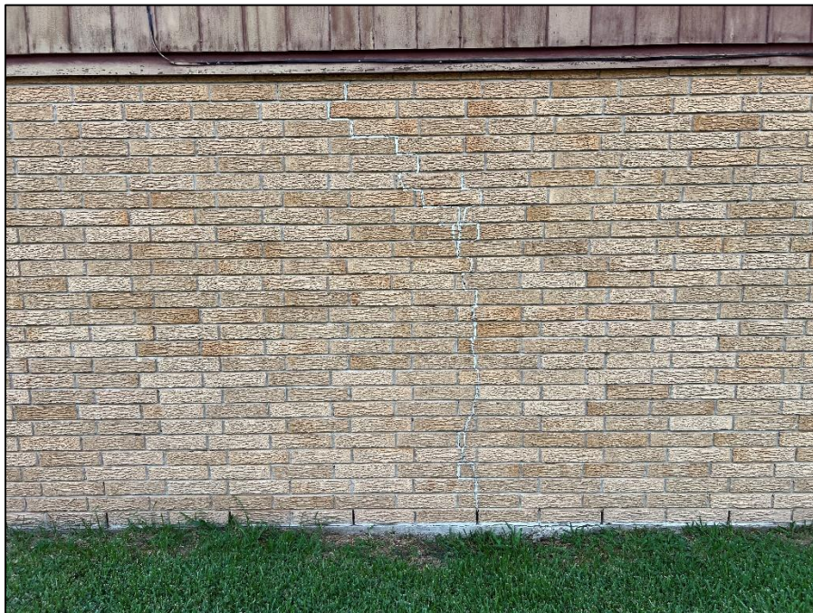
Photograph 18: Typical view of historical mortar repair at the right exterior wall of the residence.
