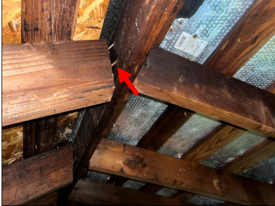
Photograph 39 : Observation of roof rafters that have been detached from the ridge board.
