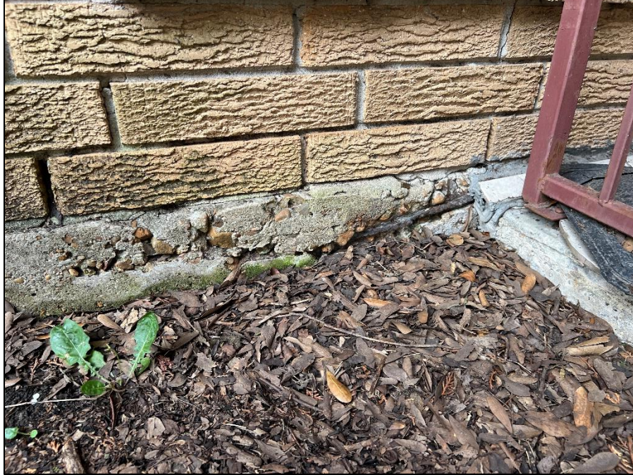
Photograph 7: Observation of concrete spalling due to the corrosion of embedded reinforcing steel at the edge of the exterior foundation grade beam.
