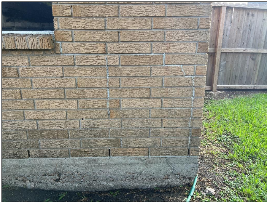
Photograph 16: Typical view of historical mortar repair.
