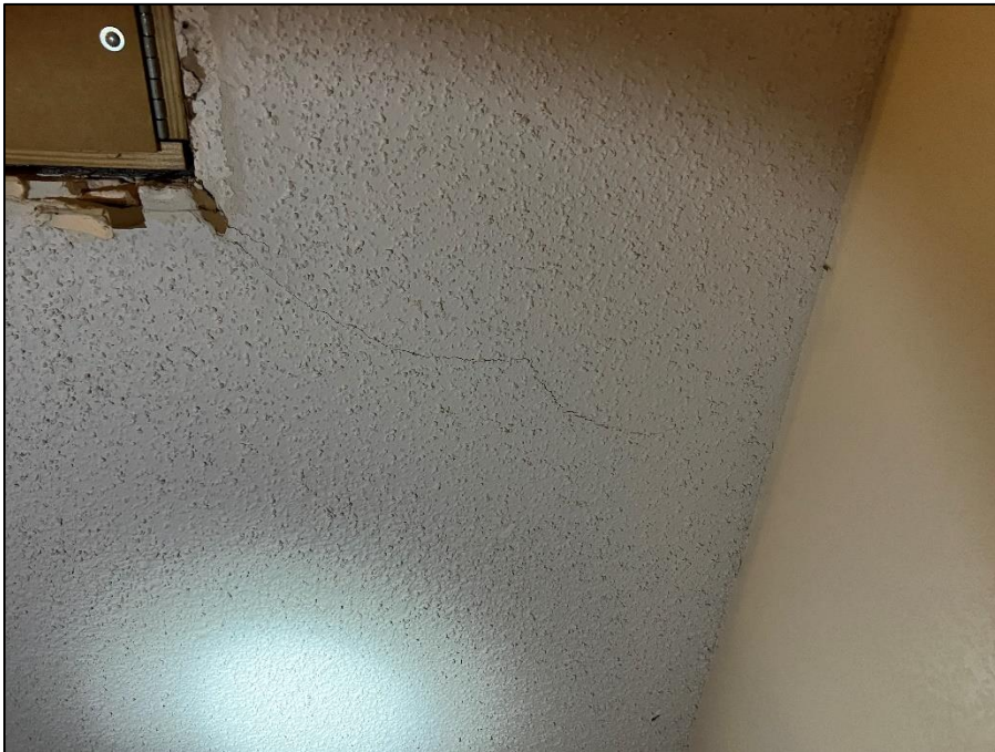
Photograph 22: Typical view of ceiling displaying drywall cracking extending from the attic access.
