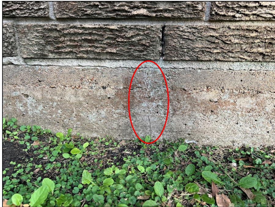
Photograph 14: Typical view of cracking on the exterior perimeter foundation grade beam at the left of the residence.
