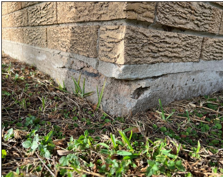
Photograph 6: Typical view of concrete corner spalling due to the corrosion of embedded reinforcing steel at the edge of the exterior foundation grade beam.
