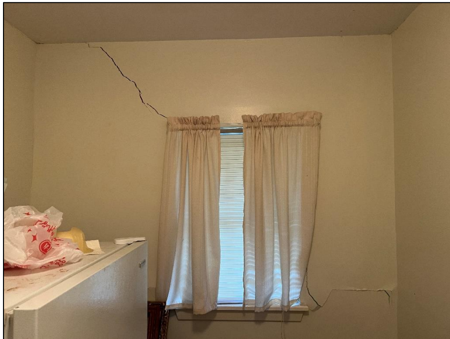
Photograph 38: Typical view of rear exterior wall of the laundry room displaying drywall cracking extending from the window header and windowsill.
