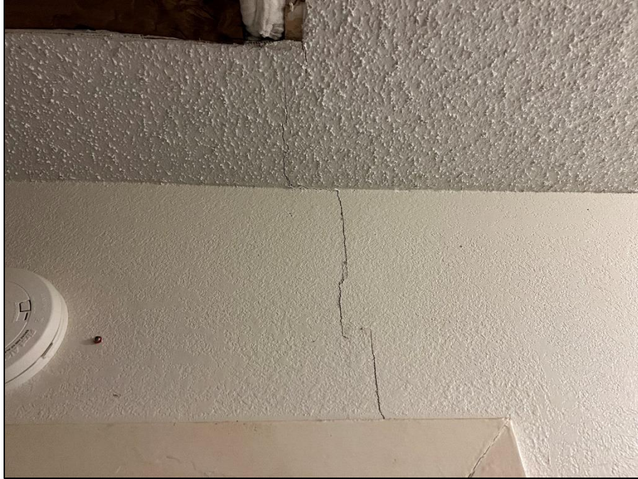
Photograph 21: Typical view of interior wall of the hallway ( adjacent to center bedroom ) displaying drywall cracking extending from the door header.
