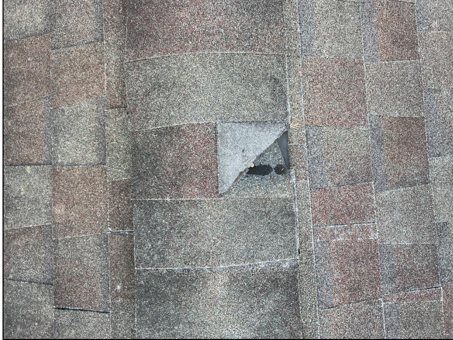
Photograph 43: Typical view of damaged, missing, and/or torn asphalt ridge caps on roof.
