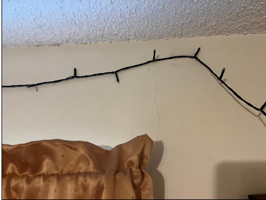
Photograph 27: Typical view of front exterior wall of the front left bedroom displaying drywall cracking extending from the window header.
