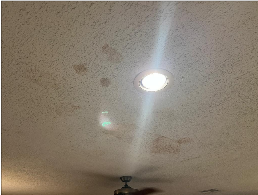
Photograph 36: Typical view of ceiling displaying moisture staining in the converted garage.
