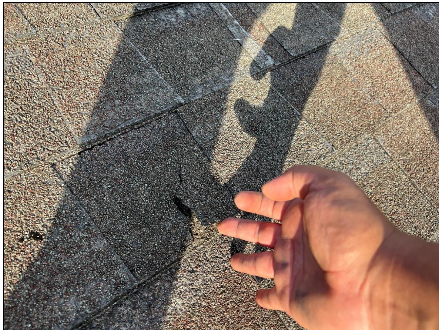
Photograph 46: Typical view of damaged, missing, and/or torn asphalt shingles on roof.
