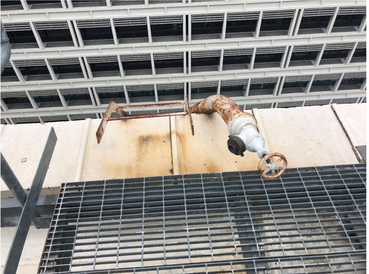
Photo 3: Top view of inoperable fire escape.
