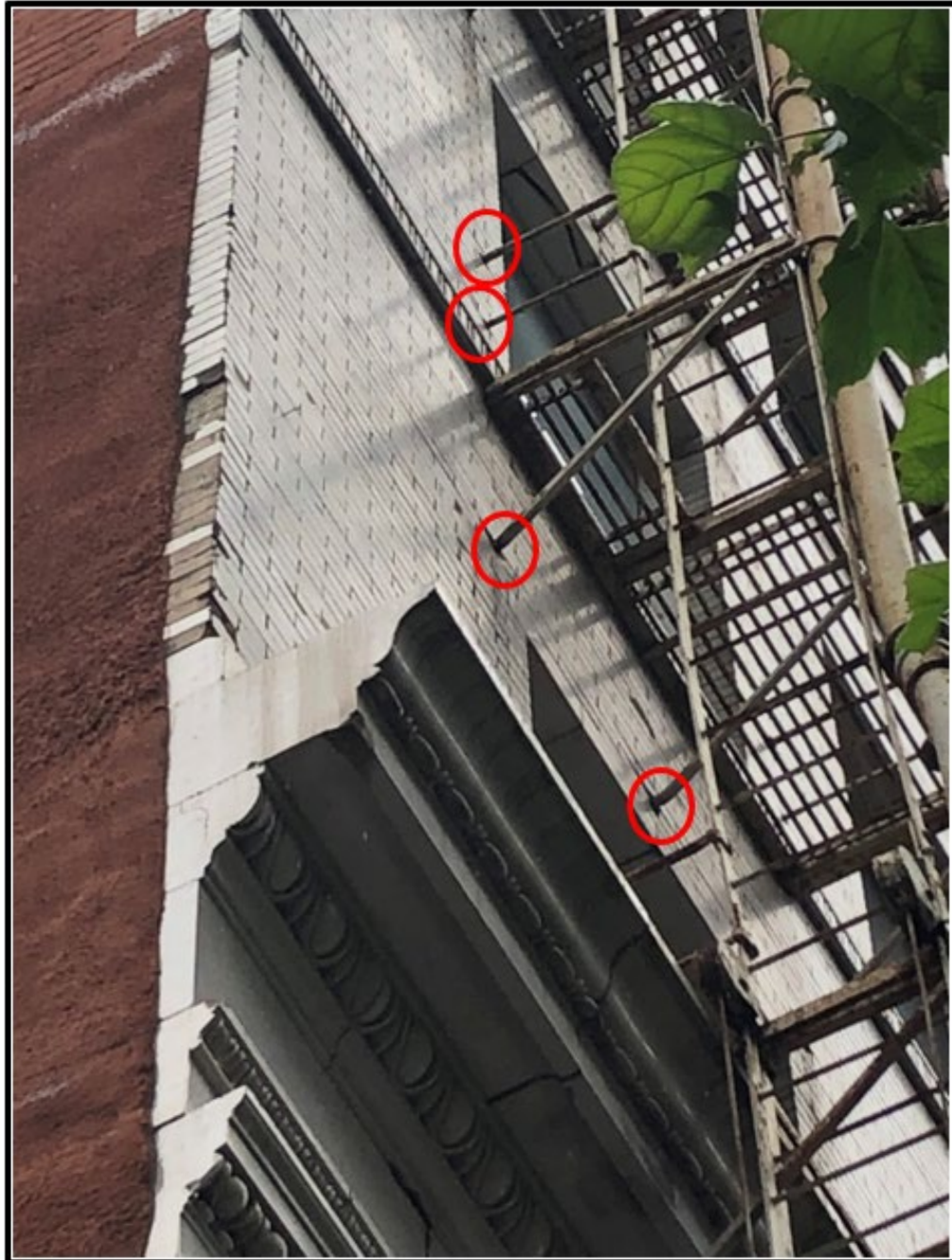
Photo 5: Representation of areas where the brick will be removed and replaced with a matching brick unit. A mortar sample will be sent in to match the existing mortar.
