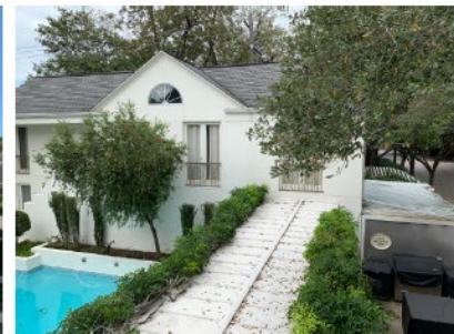
EXISTING SHINGLE ROOFING ON DETACHED GUEST QUARTERS, WHITE STANDING SEAM METAL ROOFING ON GARAGE & COVERED WALKWAY.
