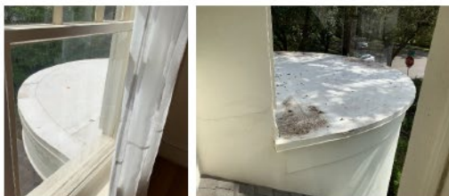
EXISTING MEMBRANE ROOFING ON 1980s ADDITIONS LEFT: OVER FRONT ENTRY, RIGHT: CURVED ADDITION
