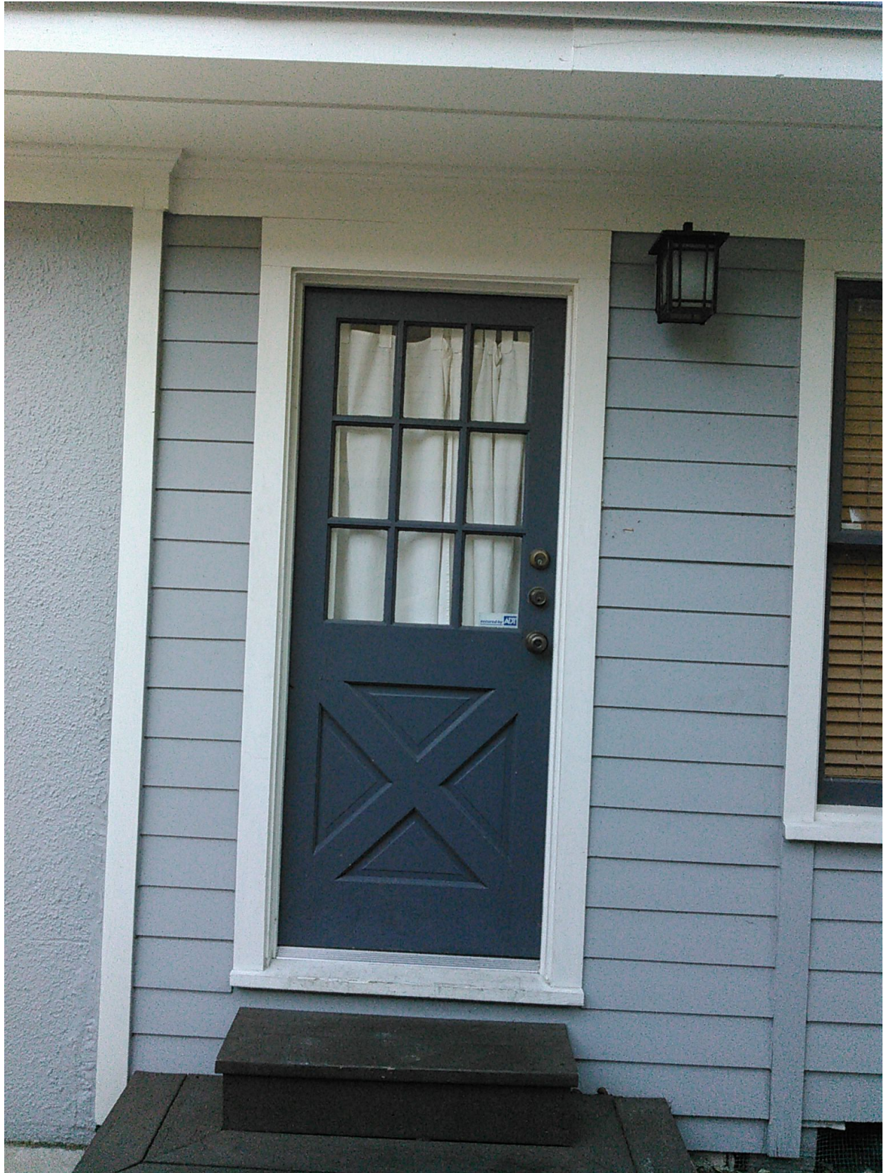
West side kitchen door showing stucco to siding transition at original to previous addition location.
