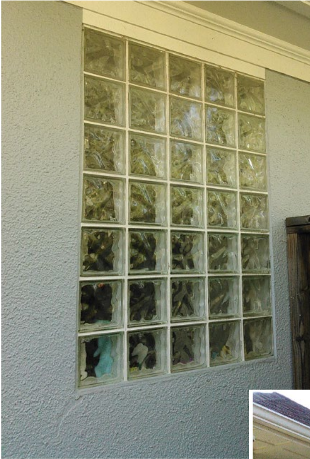
East side non-historic bathroom window to be replaced.
