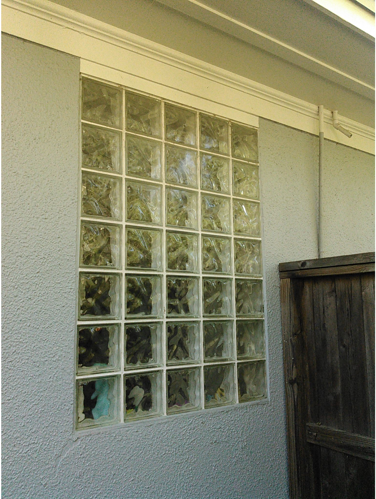
East side non-historic bathroom window to be replaced.
