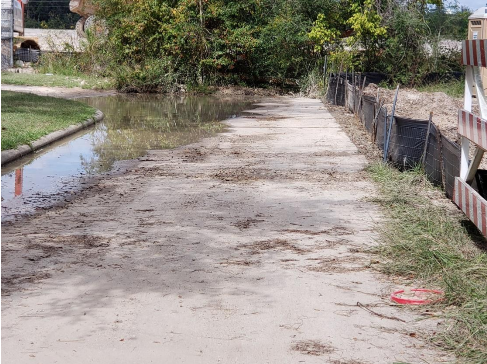
Remove Silt from Fair Grove Drive Driveway Area
