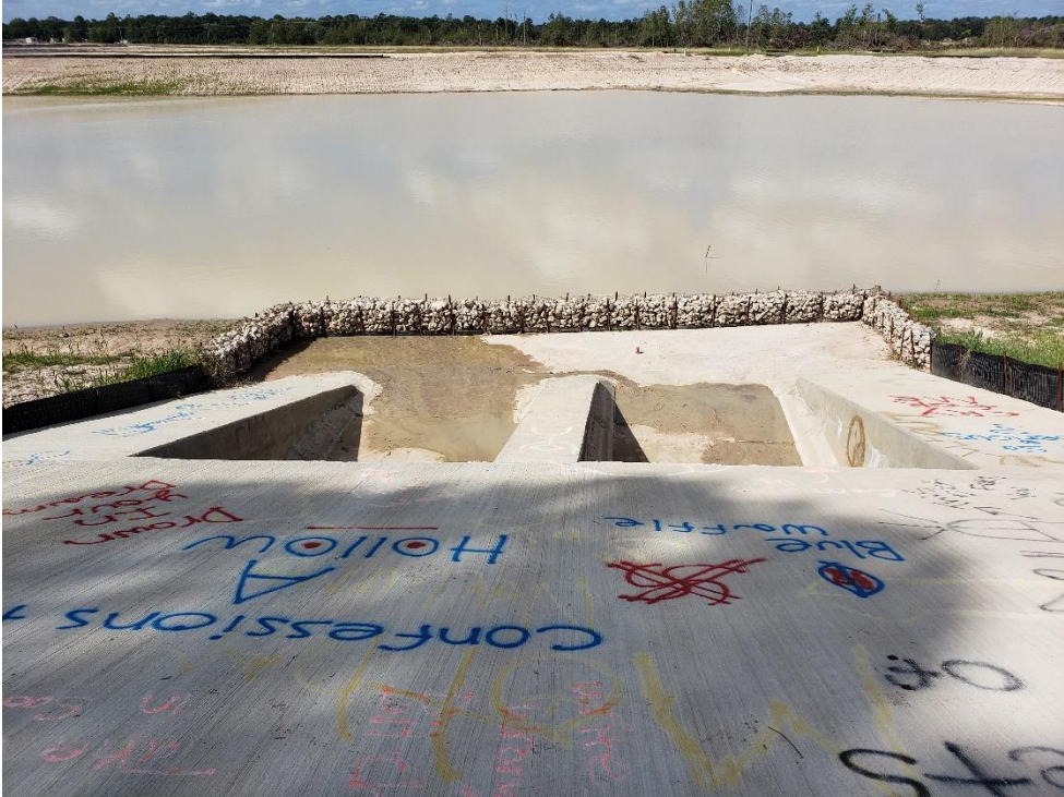
Outfall Structure on Detention Pond #1 Note: Add BMP's to reduce sediment migration
