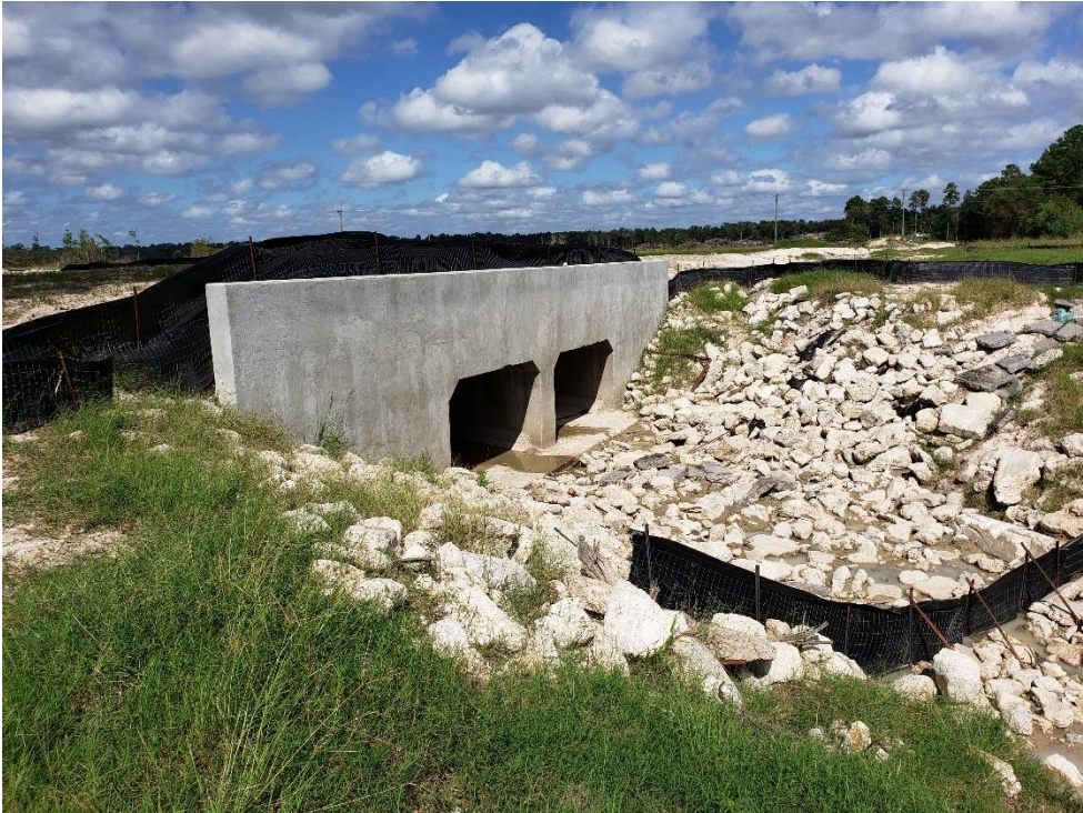
Outfall Structure's Discharge to Taylor Gulley Note: Add BMP's to reduce sediment migration
