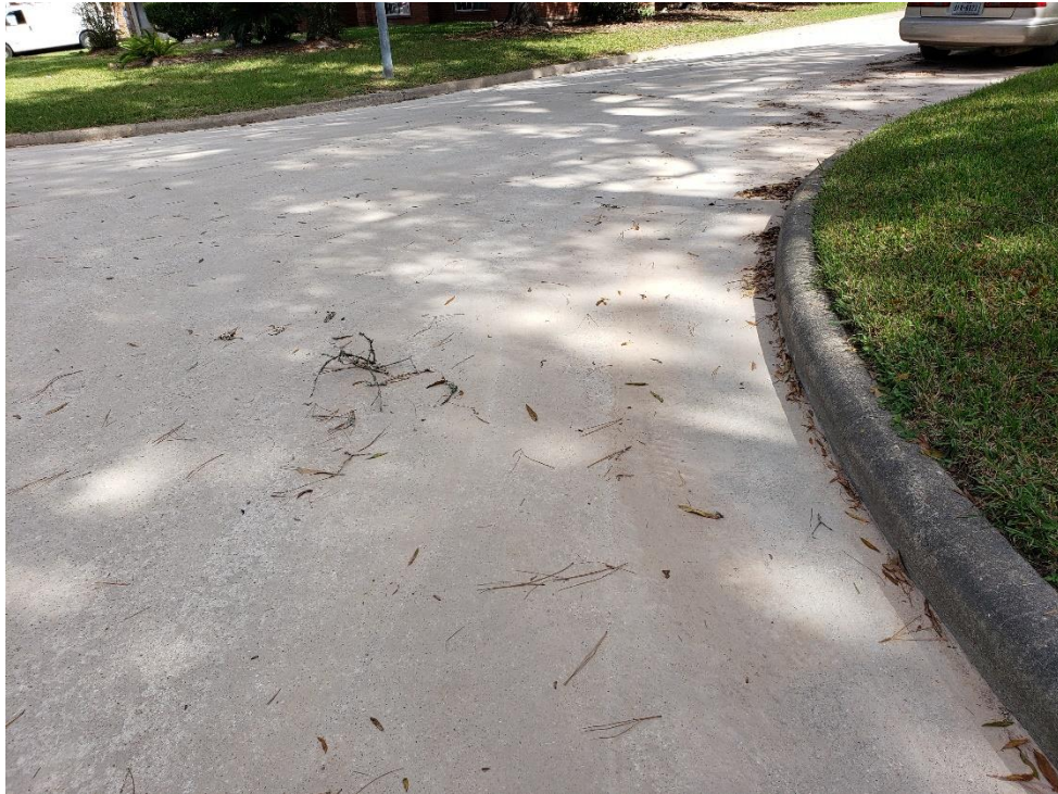
Light Sediment at Village Springs Drive and Creek Manor Drive
