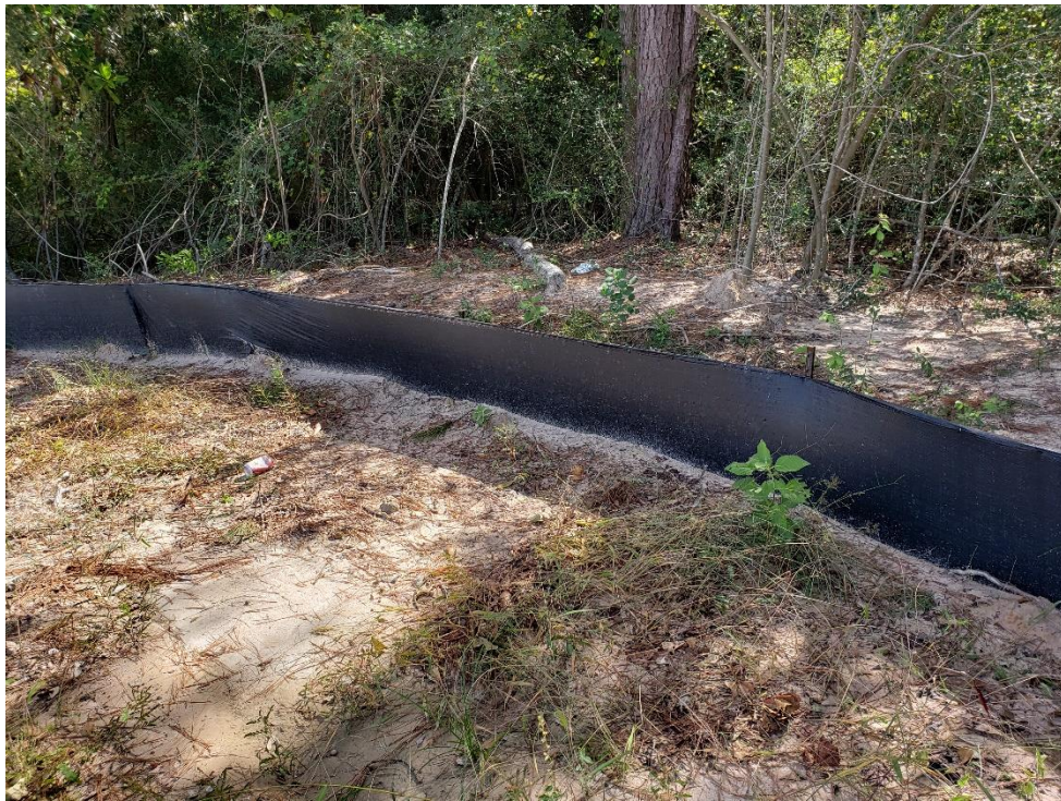
Well Maintained Silt Fencing
