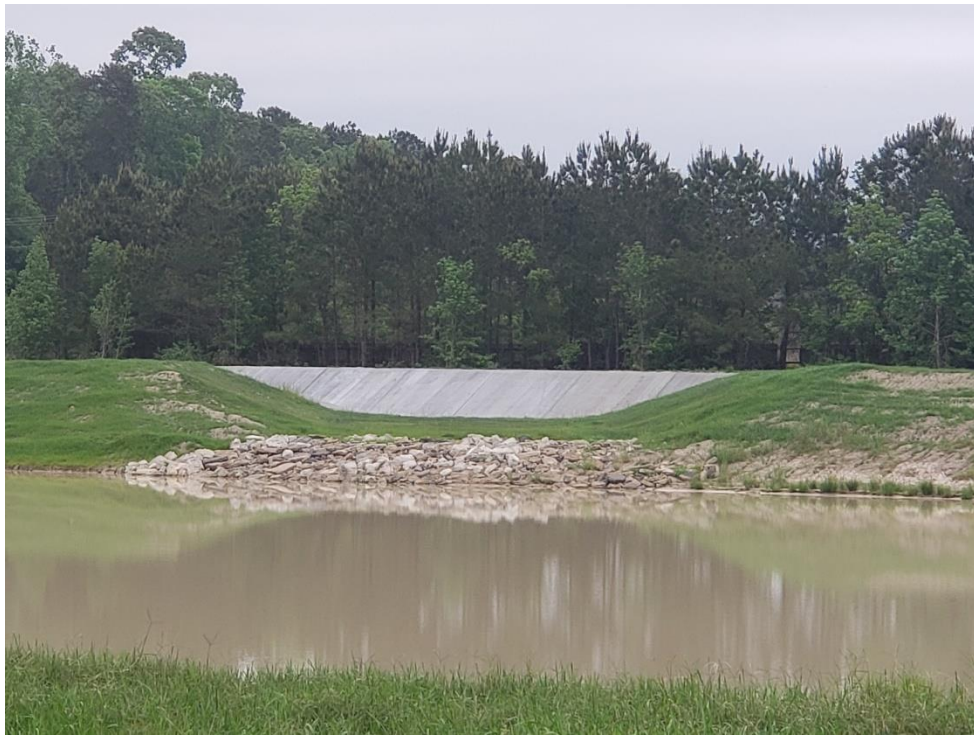
View of Overflow from Montgomery County Flood Control Ditch to Detention Pond #1
