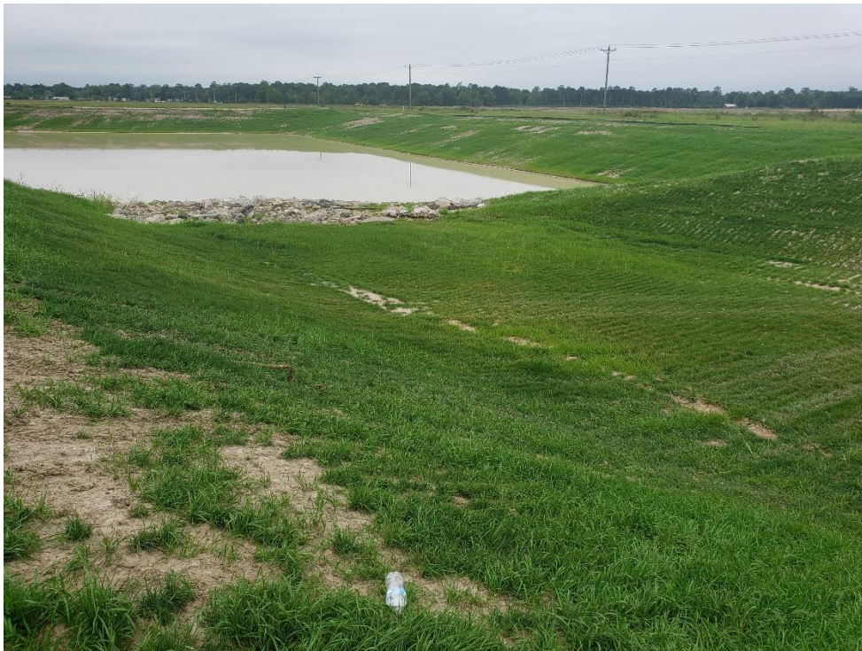
Overflow from Montgomery County Flood Control Ditch to Detention Pond #1 Note: This area has been re-stabilized with Hydro-Mulch
