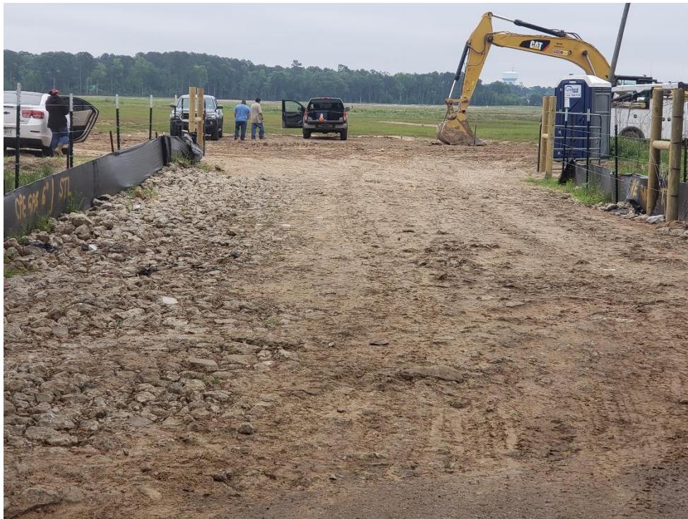
View of Construction Entrance on Webb Road Note: Light tracking and new gates
