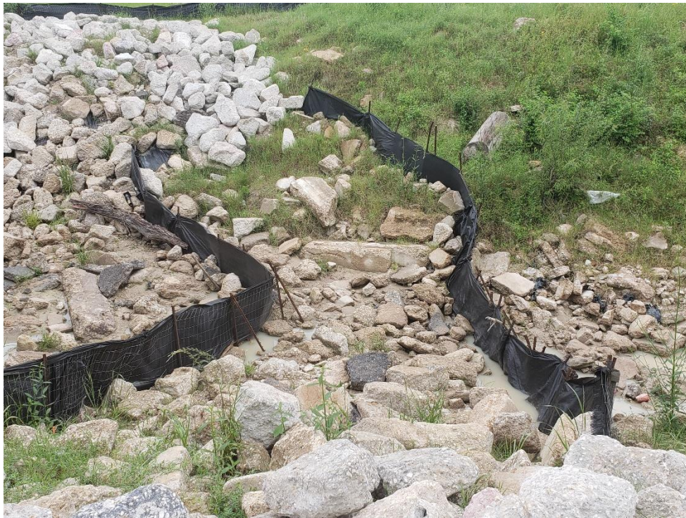
View of Outfall of Detention Pond #1 to Taylor Gulley Note: Silt fencing has been replaced
