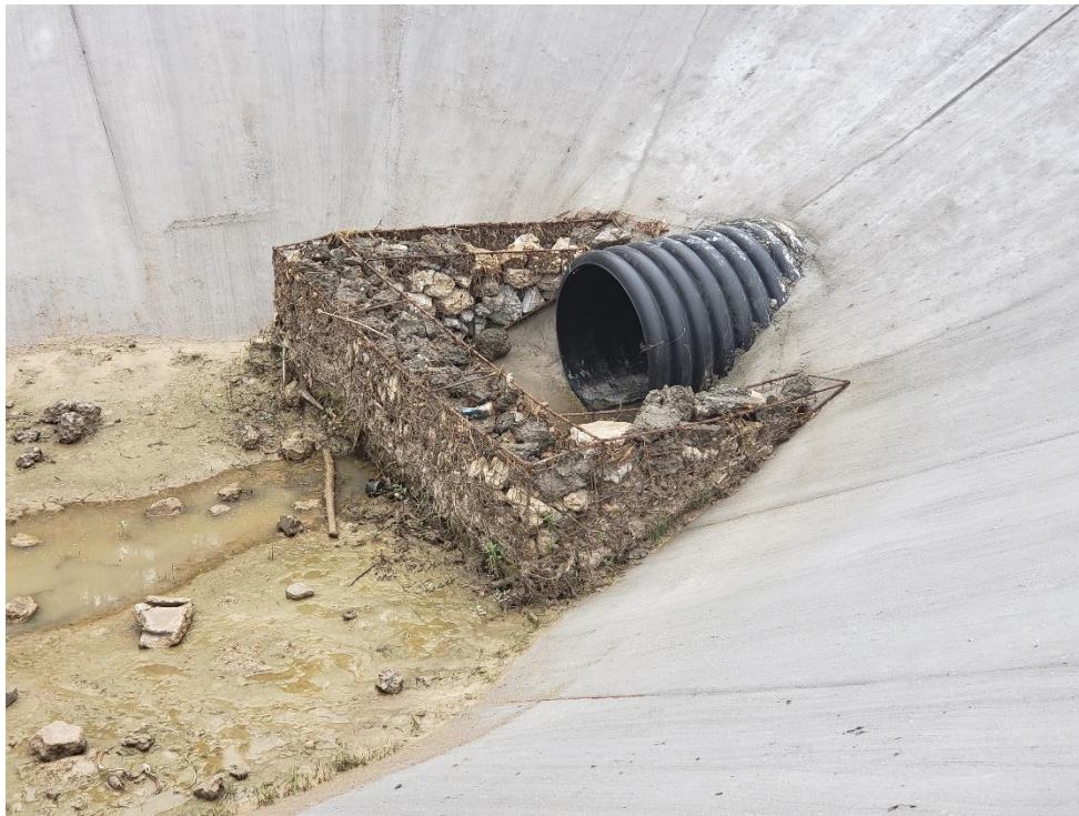
View of Upstream Outfall Structure from Montgomery County Flood Control Ditch to Taylor Gulley
