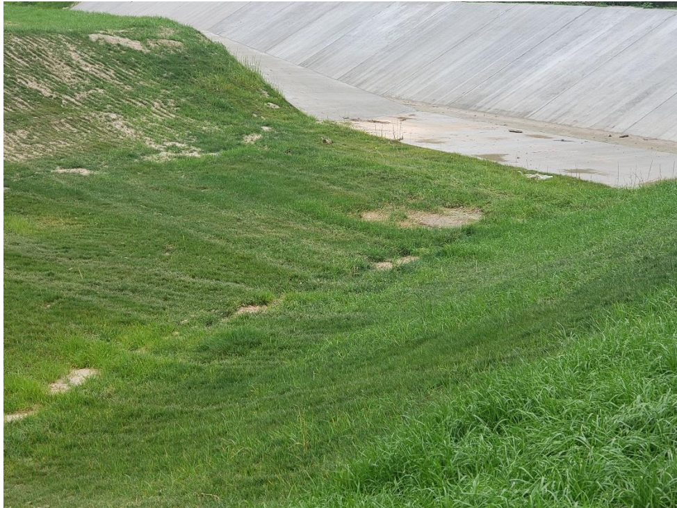
Overflow from Montgomery County Flood Control Ditch to Detention Pond #1 Note: This area has been re-stabilized with Hydro-Mulch
