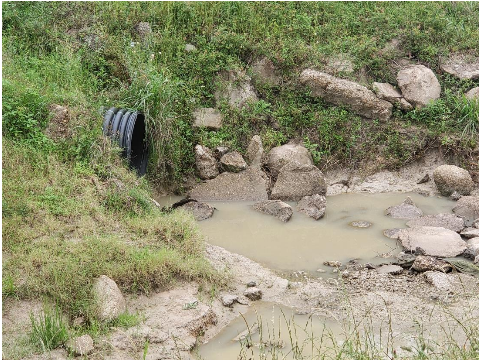
View of Montgomery County Flood Control Ditch Outfall to Taylor Gulley Note: No discharge
