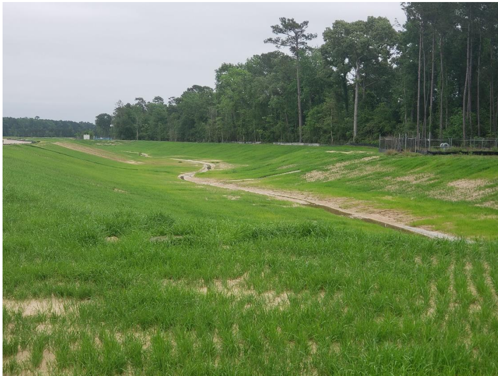
View of Detention Pond #2 Looking East Note: Grass seeds have germinated and are thriving
