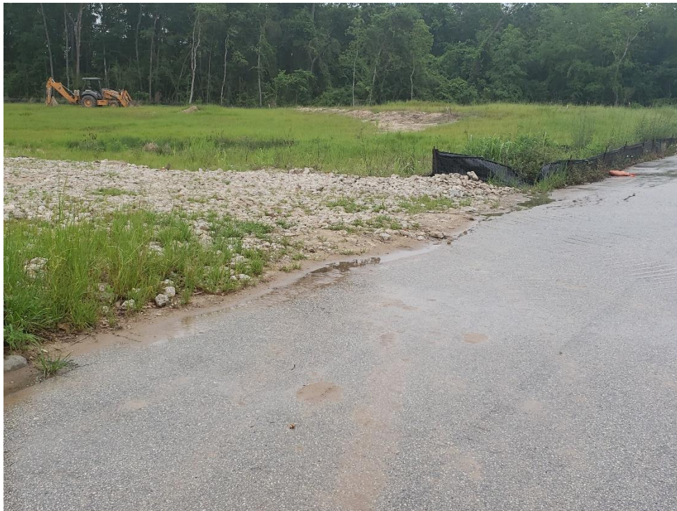
View of Construction Site Entrance on Woodland Hills Drive Note: Light tracking
