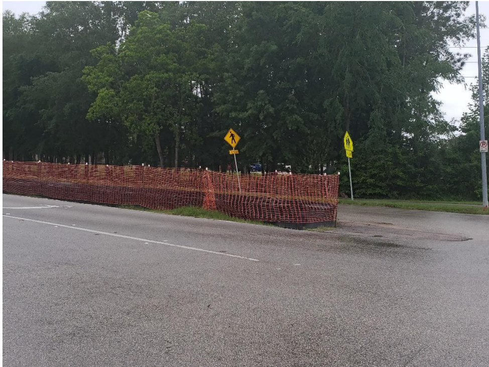
Median Protection on Woodland Hills Drive
