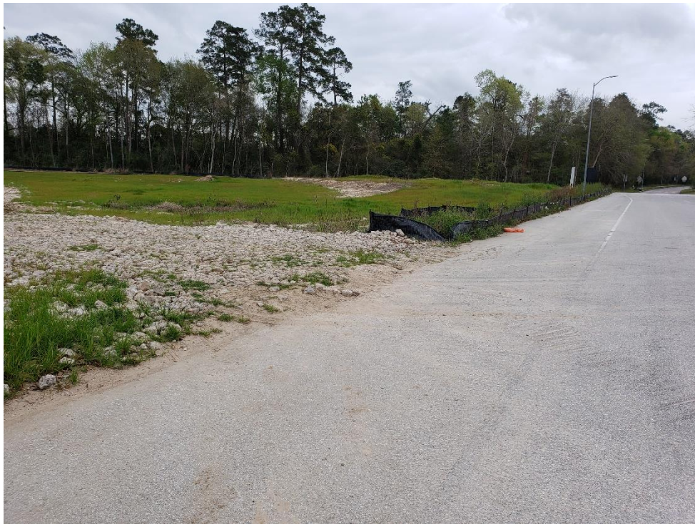
View of Construction Site Entrance on Woodland Hills Drive Note: Moderate to light tracking
