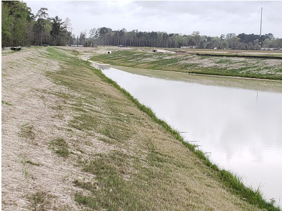
Berm between Detention Pond 1 and 2 Note: Detention pond #1 slopes are dressed and partially stabilized with hydro-mulch
