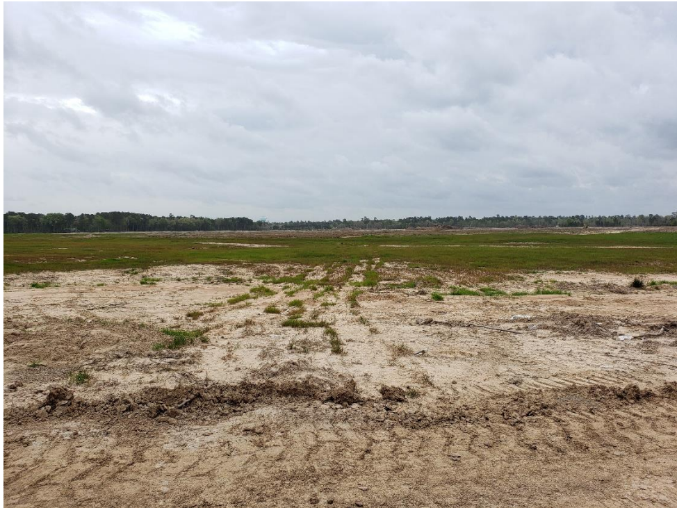
View of Northern Clear-cut Area Looking Southeast Note: Trees and brush have been chipped and piled
