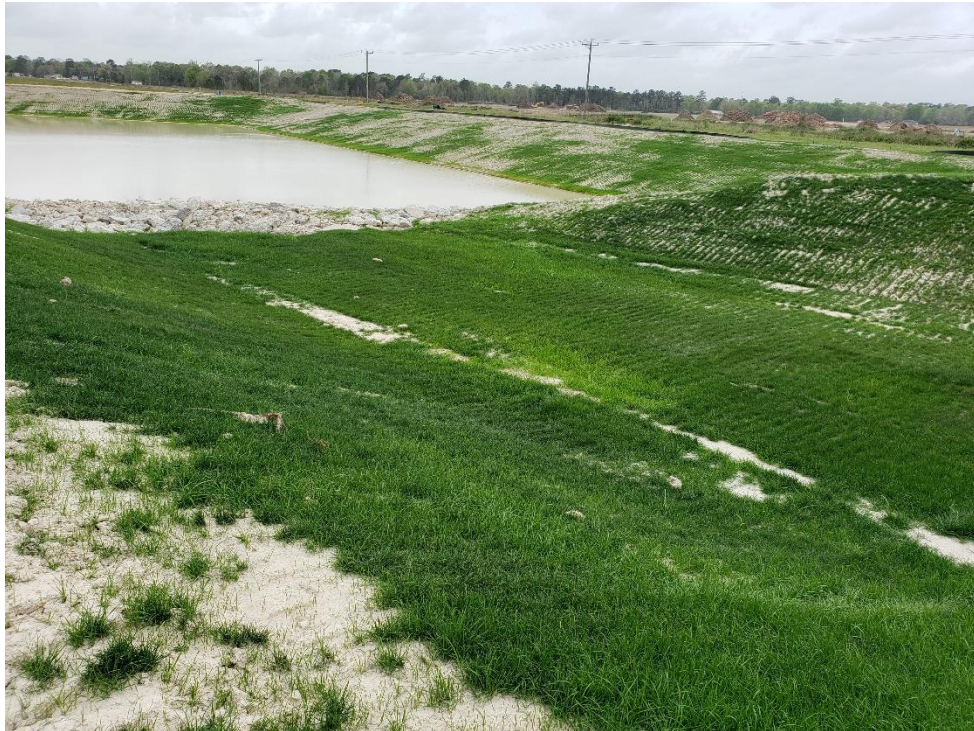
View of Overflow from Montgomery County Flood Control Ditch to Detention Pond #1 Note: This area has been re-stabilized with Hydro-Mulch
