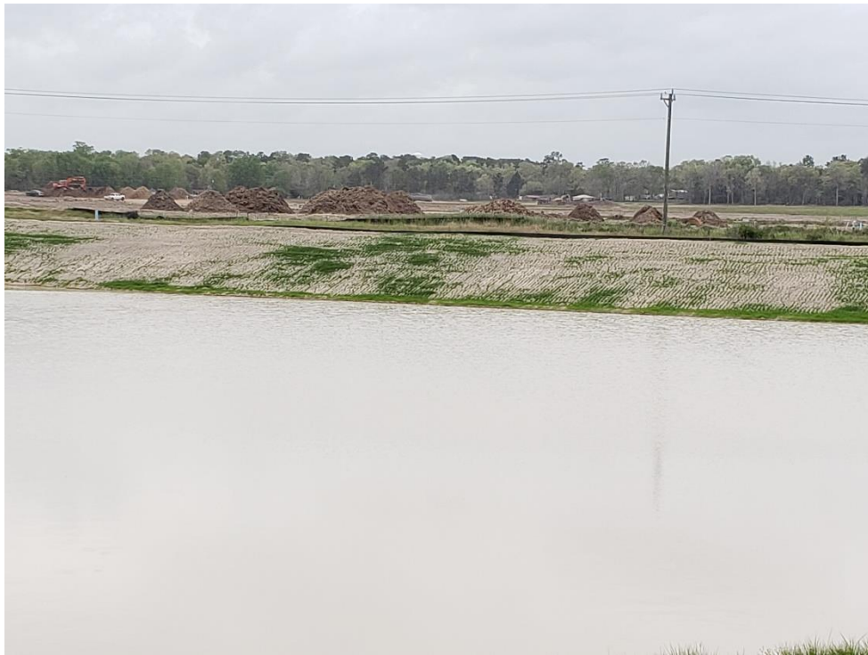
Detention Pond #1 Side Slopes are Dressed and Stabilized with Hydro-Mulch Note: Hydro-Mulch is beginning to germinate
