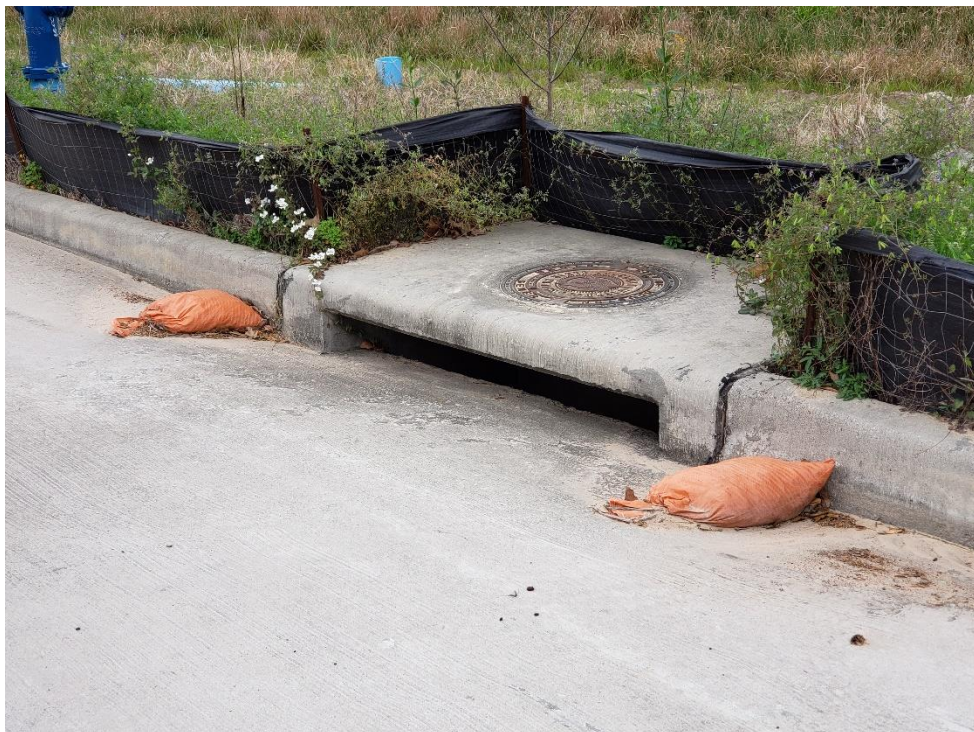
Inlet Protection on Woodland Hills Drive
