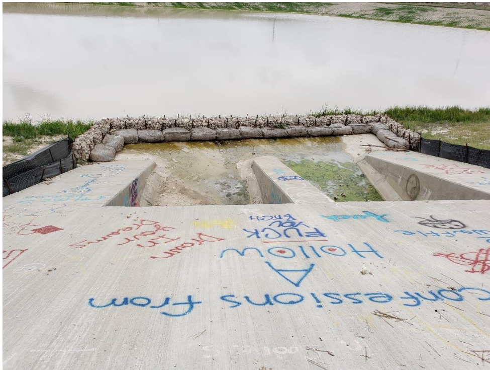
View of Upstream Outfall Structure from Detention Pond #1 to Taylor Gulley Note: Hay bales are in place and well maintained
