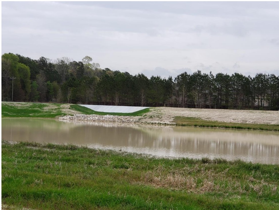
View of Overflow from Montgomery County Flood Control Ditch to Detention Pond #1 Note: This area has been re-stabilized with Hydro-Mulch
