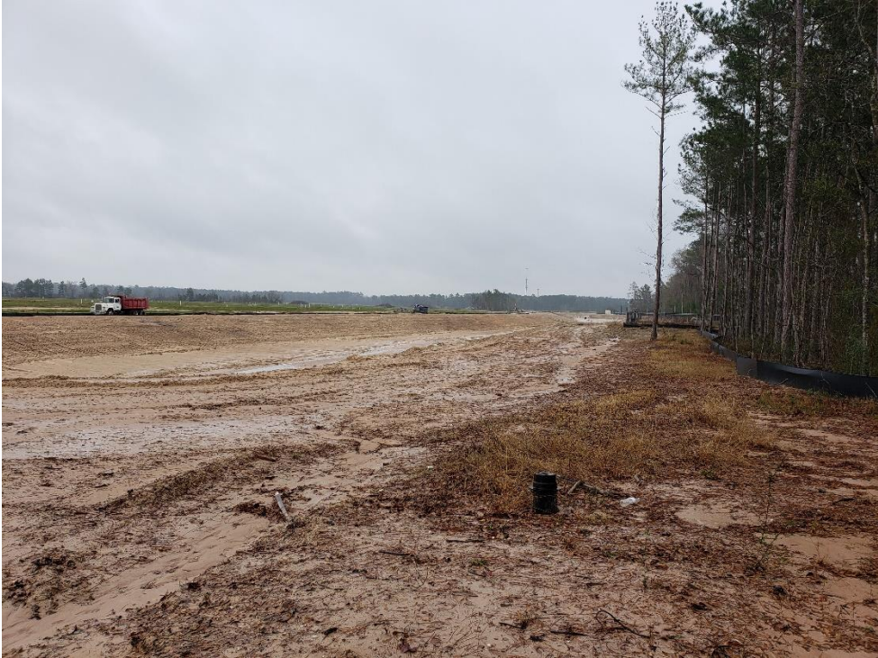
View of Detention Pond #2 Looking East Note: Detention pond has not been stabilized
