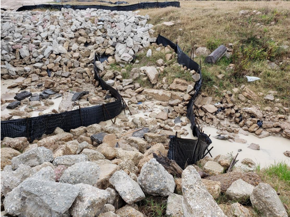
View of Outfall of Detention Pond #1 to Taylor Gulley Note: Silt fences are well maintained
