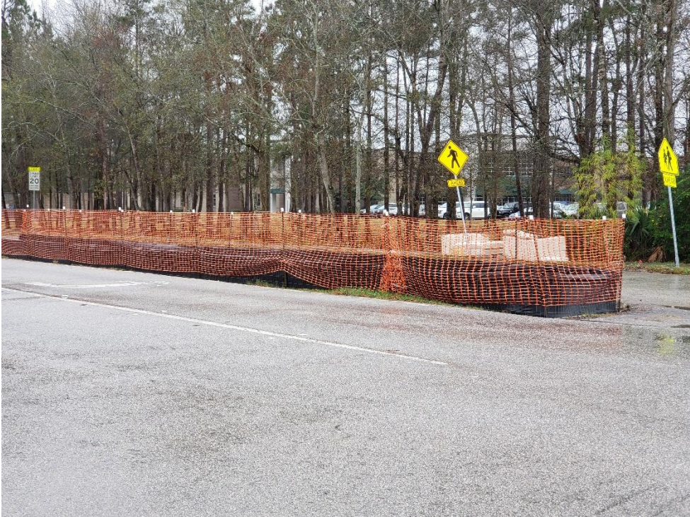
Median Protection on Woodland Hills Drive
