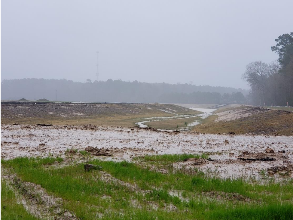
Detention Pond #1 Side Slopes are Dressed but Require Stabilization
