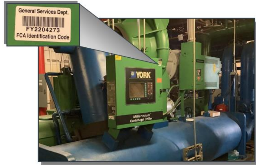
▲ Figure 1: Tagged Centrifugal Chiller #2 at Jesse Jones Central Branch Library
