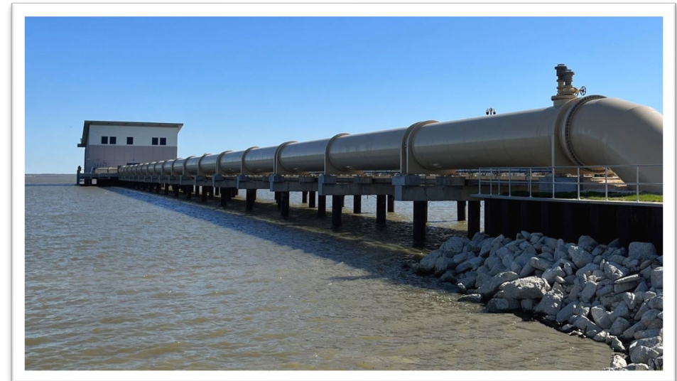
Northeast Water Purification Plant Intake Pump
