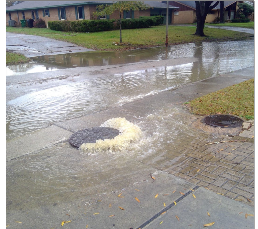
Sanitary Sewer Overflow ( SSO )
