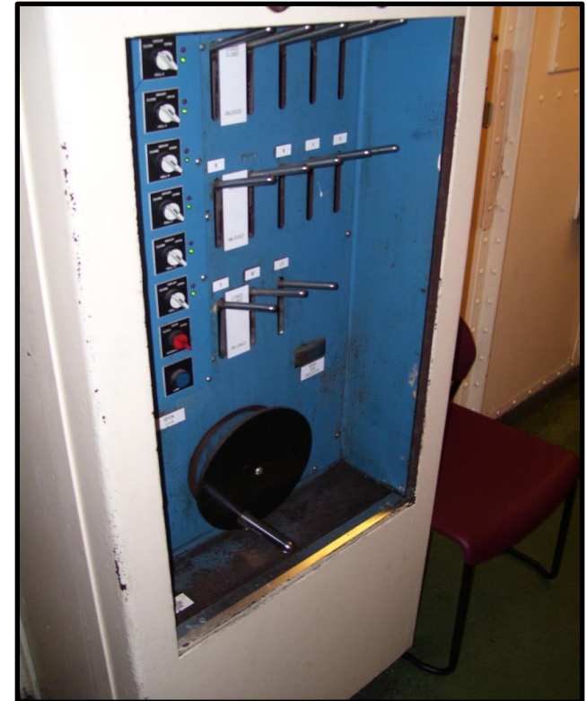
The jail door operating system is outdated.
